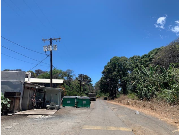
Photo 1: View facing north of pole-mounted transformers located along Olowalu Village Road.
