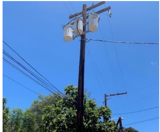
Photo 4: View facing northwest of pole-mounted transformers located along Olowalu Village Road.
