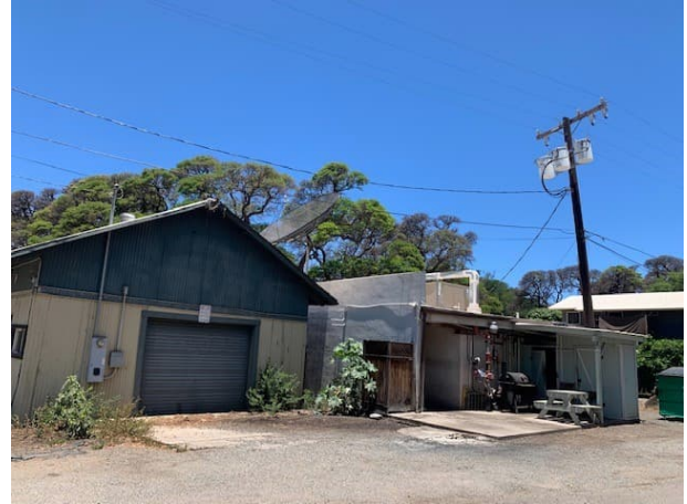
Photo 2: View facing northwest of pole-mounted transformers located along Olowalu Village Road.
