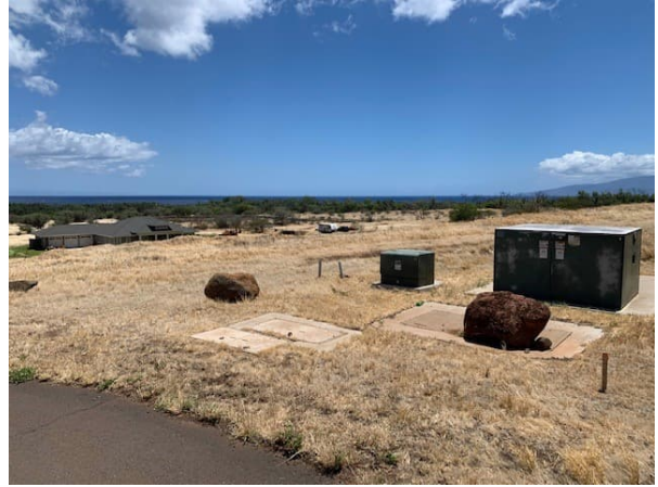
Photo 2: View facing northwest near eastern terminus of Pohaku Aeko Street. Location of Meco Pad-Mounted Transformer site listed within HEER database records.
