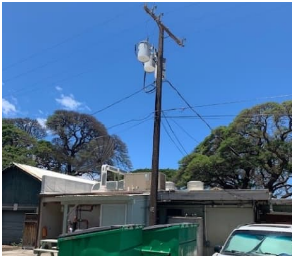
Photo 3: View facing west of pole-mounted transformers located along Olowalu Village Road.
