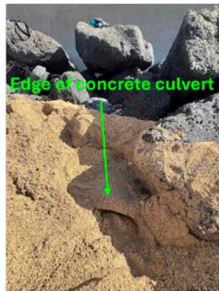
Photo depicting the sand blocking the culvert at Location 1a.
