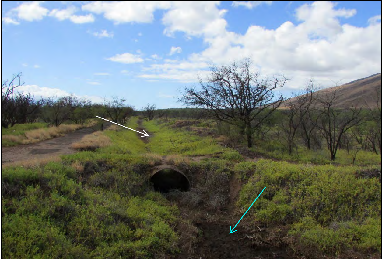
Photo 63. Culvert Connecting the North-South Ditch 7 (White Arrow) to the Hanaula Gulch (Blue Arrow)
