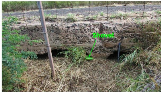
Green shovel depicted in the center of the photograph within the culvert. Ruler on the right indicated an 8 inch measurement
