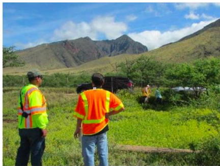
Arched culvert on the ocean side of the inner Cane Haul Road that was mostly buried and blocked with sediment.
