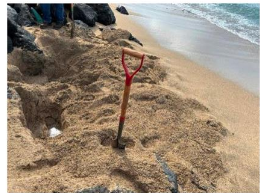
Photo depicting water ponding on the ocean side of the culvert at the existing Honoapiilani Highway.
