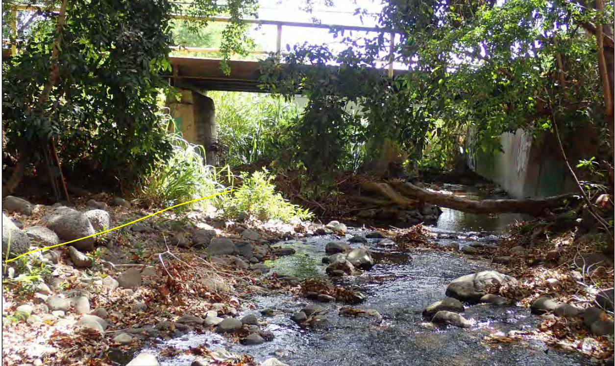
Photo 86. Location of Transect 3 At the Olowalu Stream Bridge; Sediment Staining on the Concrete Bridge Contributed to Determining the OHWM Level in this Area
