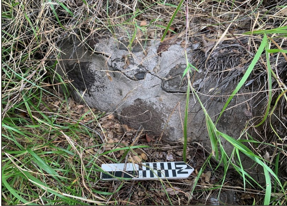
Figure 4.125. Image of the character and condition of the exceedingly common Plantation era concrete and stone infrastructure found in the region.
