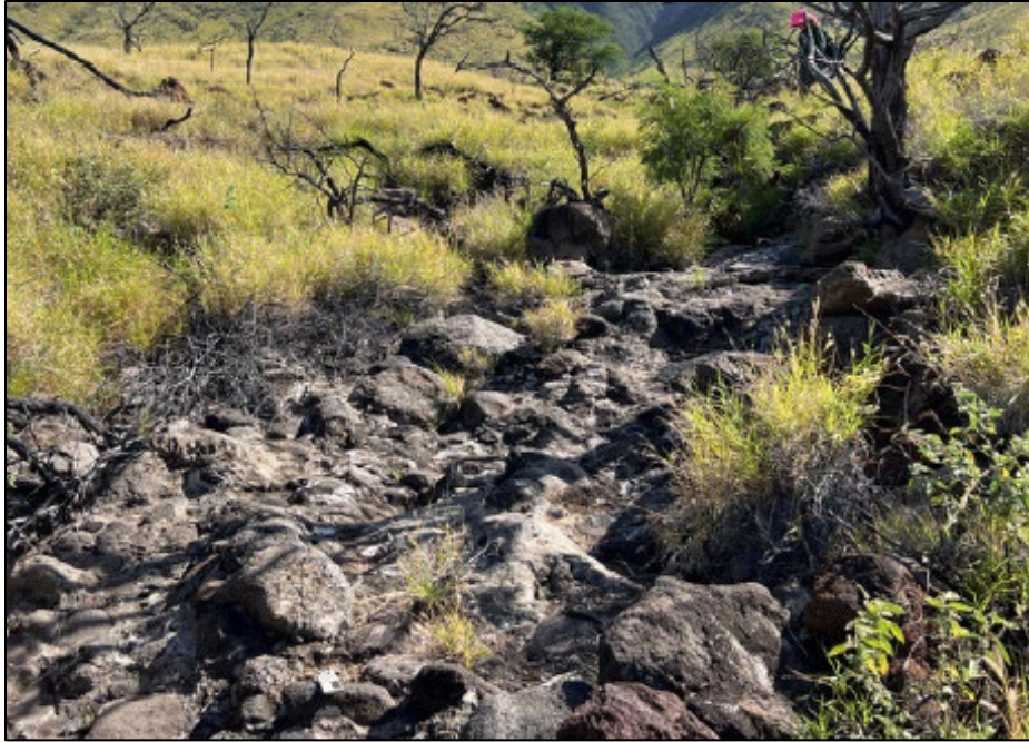
Figure 4.115. View of fire damage along flume floor.
