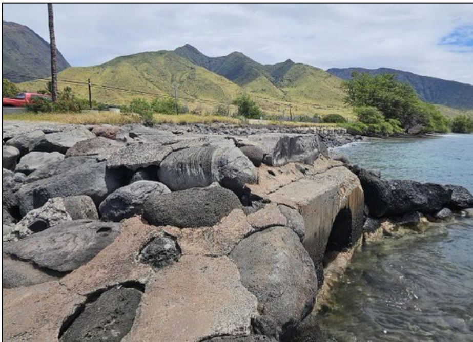
Figure 4.83. South elevation of AR 18, facing northwest; note the concrete drainage pipe emptying into the sea.
