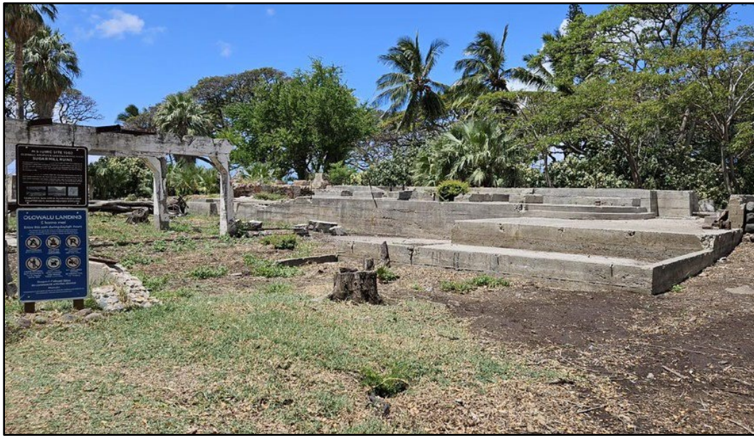
Figure 4.33 . Detail of north (front) and east elevations of extant foundation of the “12 Roller Mills” and “Molasses Tanks,” facing southwest.
