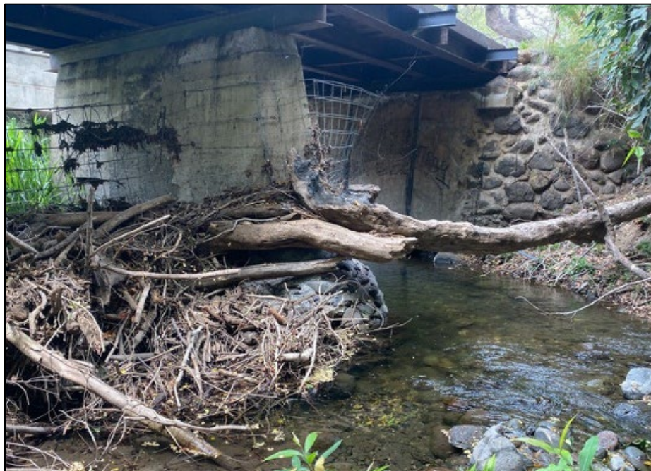
Figure 4.90. View of AR 20 superstructure and substructure, facing west; note the stream debris and deteriorated pier.
