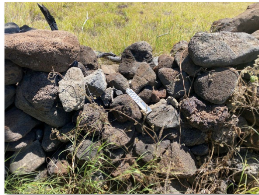
Plate 34. AA2216-073, closeup of wall construction with coral in it, view to northwest.
