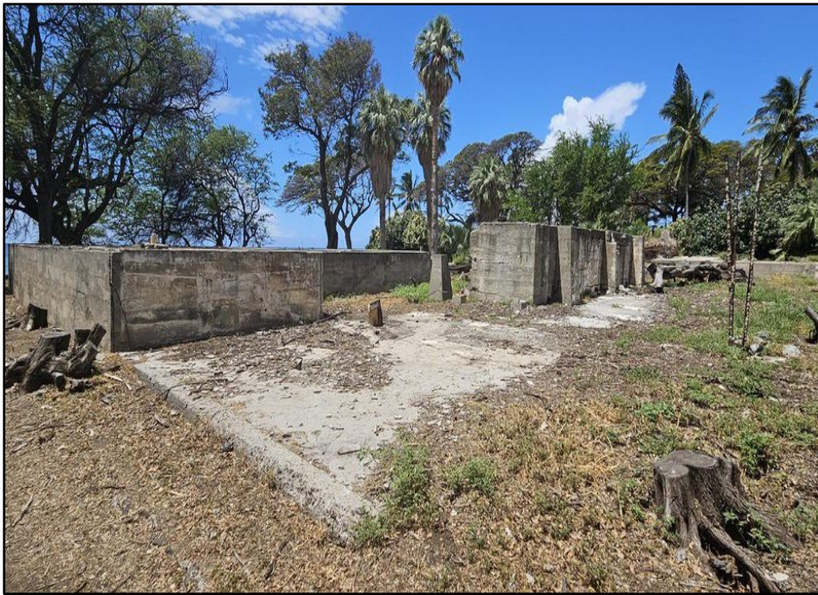
Figure 4.31 . Detail of east elevation of extant remains of “Sugar Warehouse,” facing southwest.
