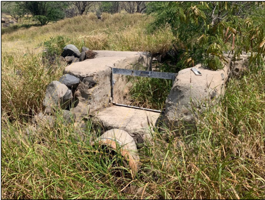
Figure 4.160. View of AF 36, facing north; note sluice gate and stacked rock exposed where concrete is eroding.
